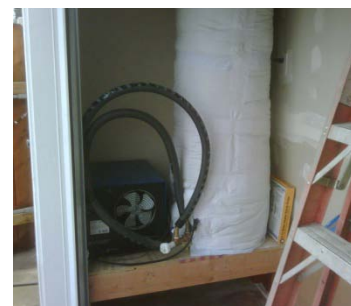
Figure 3: HPWH and Tank
