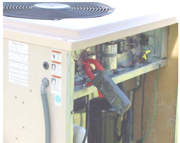
Verify Amps On All Components
