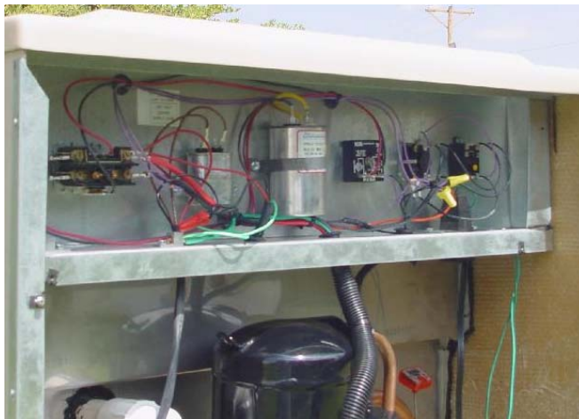
Freus Wiring Panel
