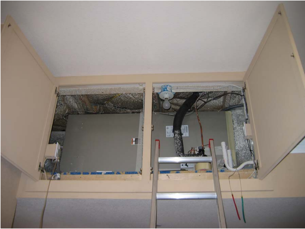
Figure 10 Air Handler Attic Access Cabinet Typical of Borrego Prototypes
